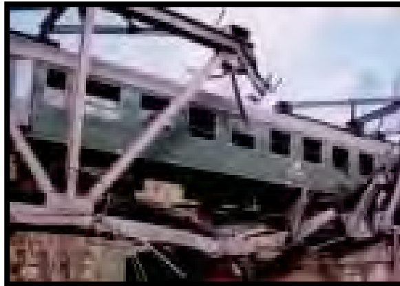
Figure 7-24. Example of a damaged rail transportation system.
